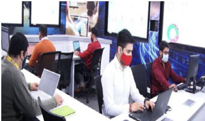
RailTel SOC at Gurugram
