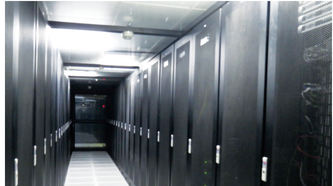
RailTel Data Center at Gurugram
