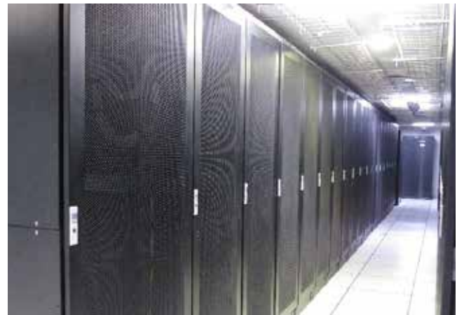
RailTel Data Center at Gurugram
